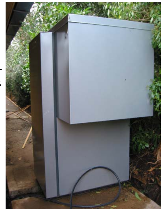
Heat collecting unit at Welburn Village Hall
